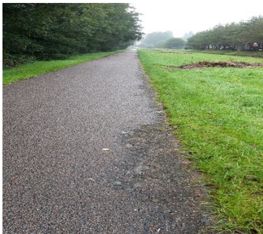
Hoge berm/afbrokkeling asfaltrand.
